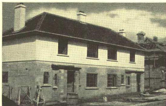
Pomphlett Gardens Housing Scheme : house nearing completion. The outer walls are of white roughcast, chimneys are white and tiles brick red.
