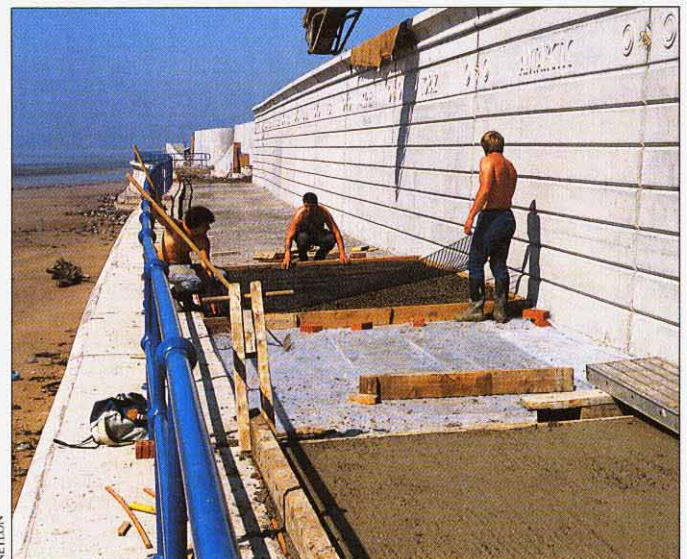
Tensar grids were used to reinforce the concrete promenade walkway at Swansea.
