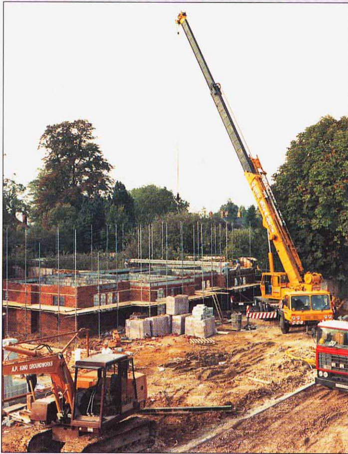
The discipline of delivery dates eliminates delays in bringing walls to first-floor level.
