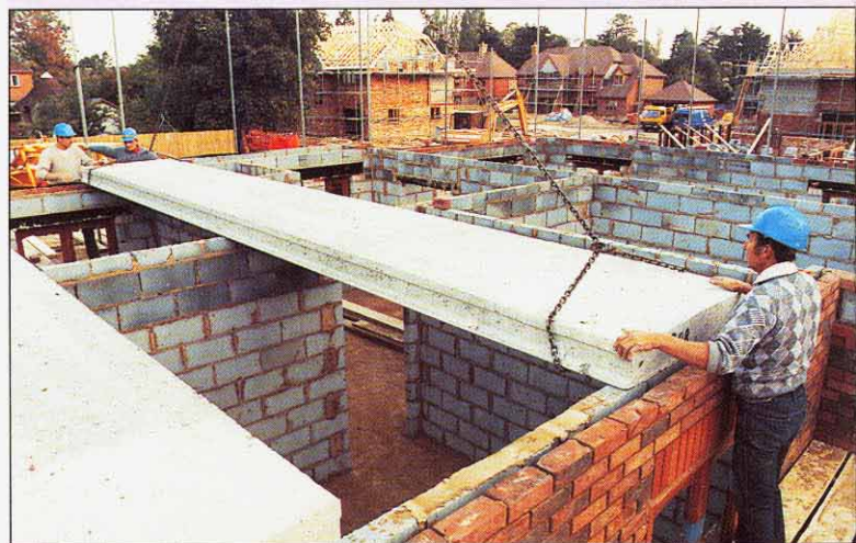
Installing the 1200 mm wide prestressed concrete floor units on a development in Maidenhead.
