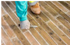
ABOVE It is vital that the joints between the boards are completely watertight
