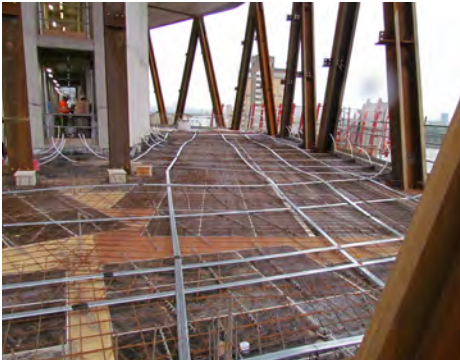
ABOVE High-strength tendons draped within a floor slab, waiting for the concrete to be poured at the Newfoundland tower, London
