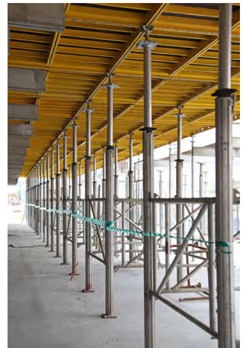
ABOVE Hunnebeck's TOPEC modular slab formwork in use at Helical Bars Fulham Wharf development in London
