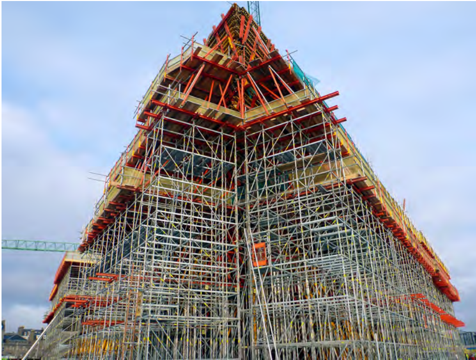
ABOVE AND LEFT The formwork for Kengo Kuma's V&A Dundee comprised 1,200 unique CNC-cut shutters, created by Peri from plywood-faced timber with a controlled-permeability liner. These were supported on a vast system of steel falsework
