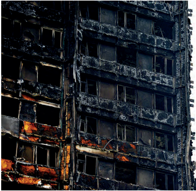
ABOVE The changes to the regulations were prompted by the Grenfell Tower tragedy in London – the worst UK residential fire since the Second World War. The rapid spread of fire was blamed on the building's exterior cladding
